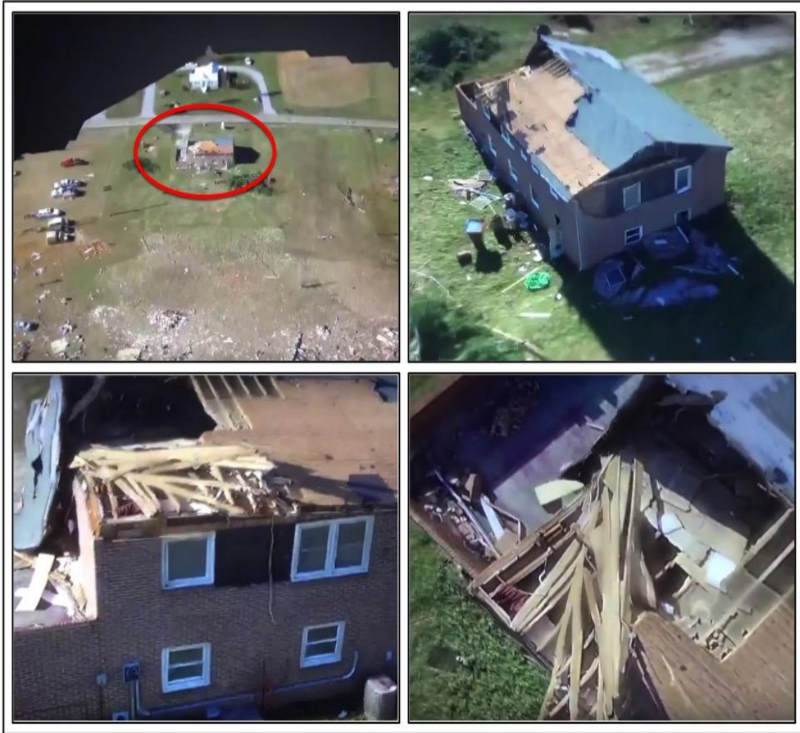
Figure 21. Computer screen captures of a textured DSM with a wide angle oblique view of an affected area (top-left), a zoomed in oblique view targeting a two-story home from multiple angles (top-right; bottom-left), and a nadir view of roof damage from the same home (bottom-right). Imagery produced by Autonomous Flight Technologies, Inc. and provided courtesy of NWS Blacksburg.
